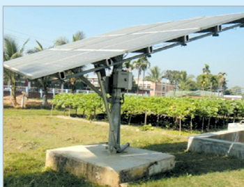
Fig. 3.13: Solar pannel installed with auto-tracker structure
